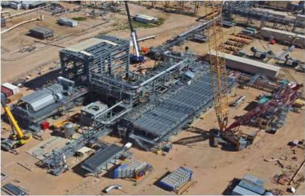
Compressor shelter and heat exchangers
