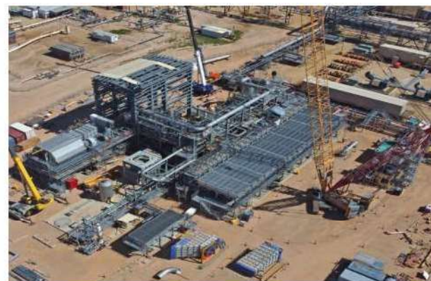
Compressor shelter and heat exchangers
